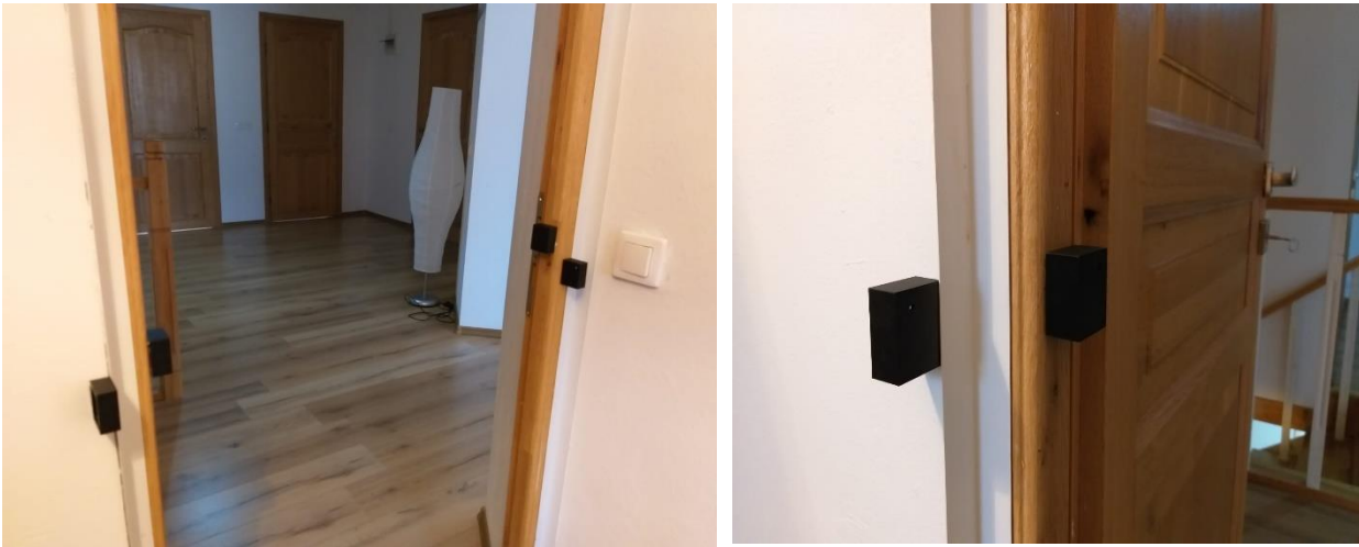
Our sensors on the door frame
